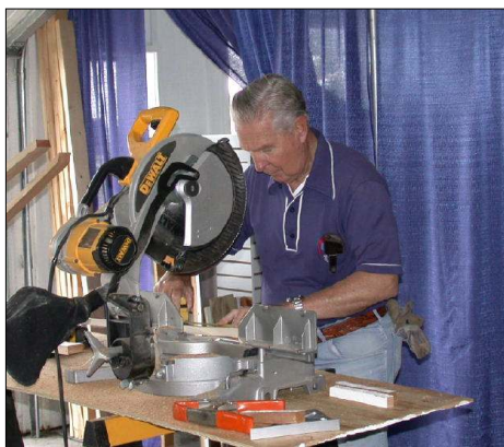
Lon Danek prepares a piece of wood trim to finish off a wall remodeling project.
