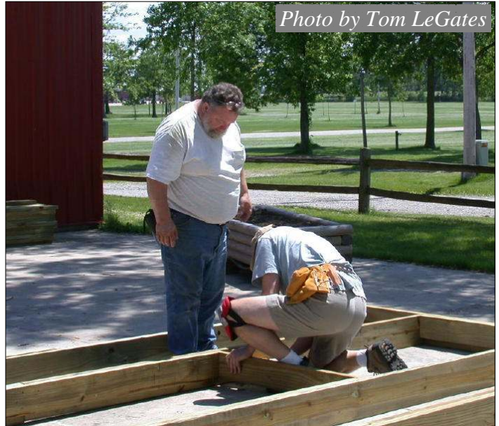
Bud Herod and Carl Geiger building the frame for the new Seaplane Base dock.
